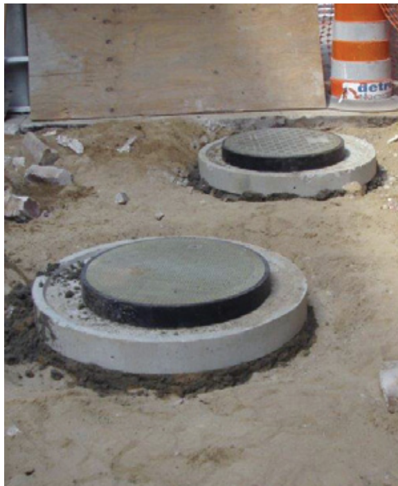
Newly installed composite manhole covers look just like the old ones, but prevent water from getting into the manhole.
