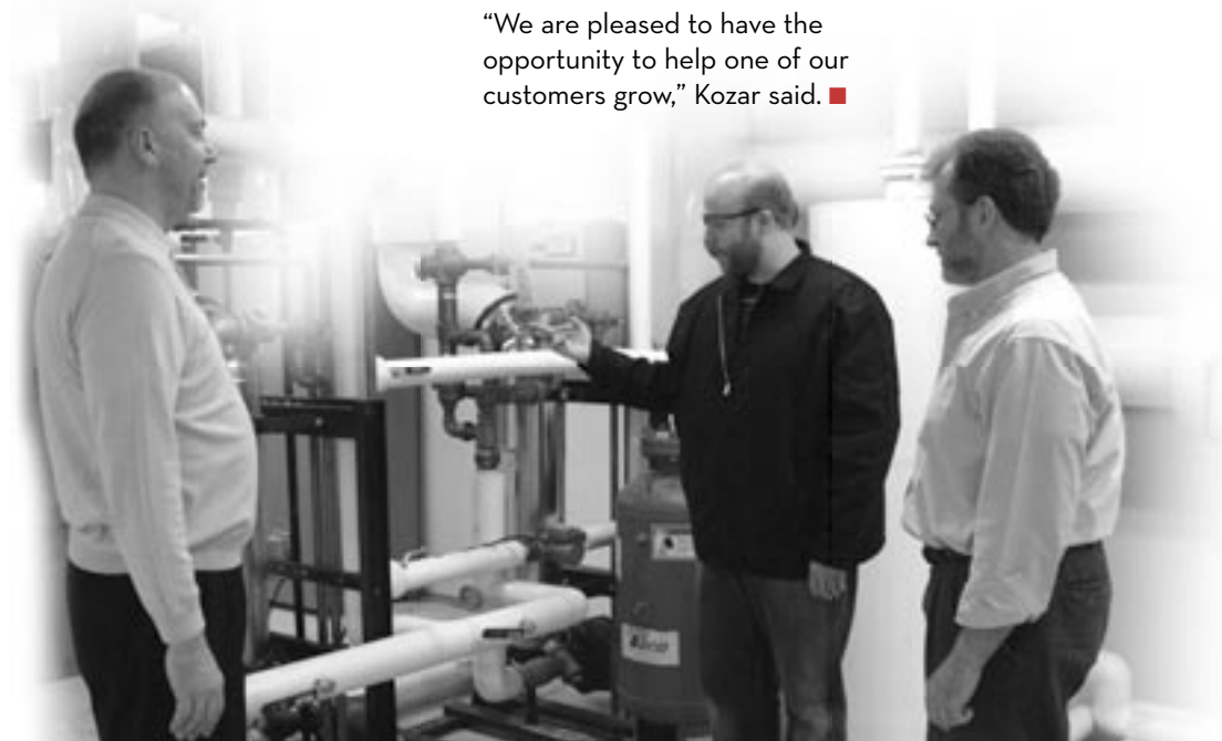
From left: John Kozar; Jeff Smigielski-McHenry, BD facilities engineer; and Lee Bowling examine a section of the company's new steam equipment.
