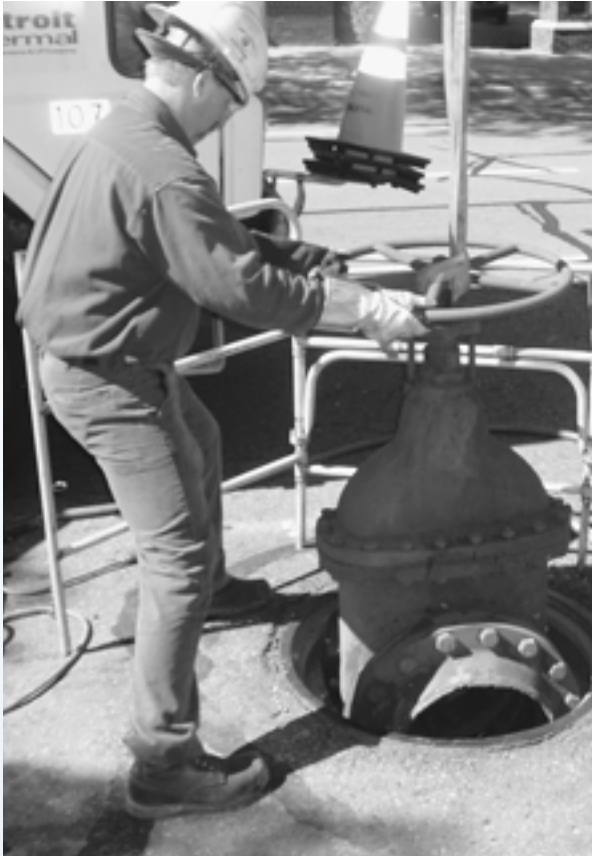
Replacing old valves has improved the efficiency of the steam distribution system.
